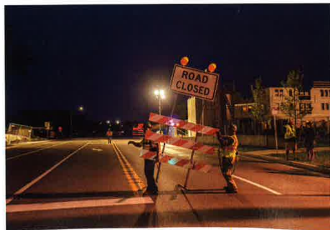
Lancaster Avenue is closed to traffic as crews work through successive nights to complete the placement of the beams for the pedestrian bridge.
