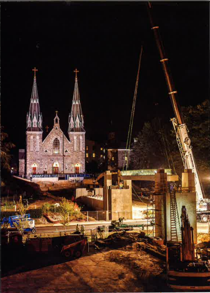
The pedestrian bridge in front of St. Thomas of Villanova Church takes shape as workers lower the center beam into position.
